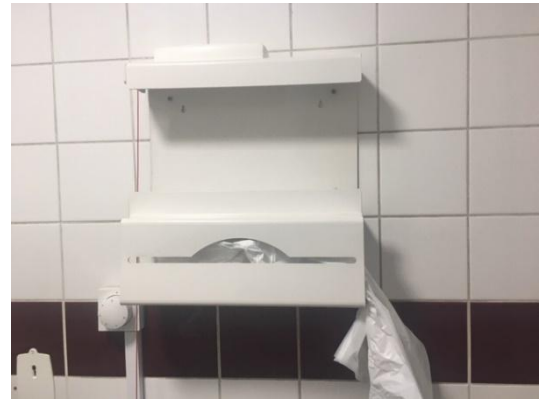
No gloves in bathroom
